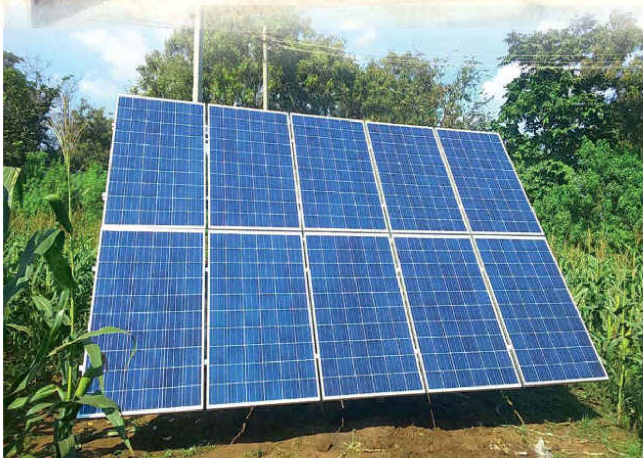
Solar Photo Voltaic (PV) Power Pumping System
