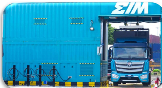
Swapping + Charging station Spare Battery Packs Charging Swapping Bay
